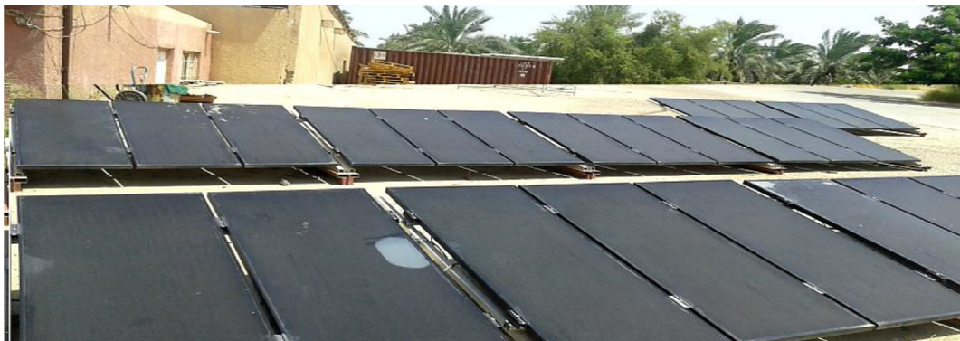
Fig. 1. CIGS solar PV system.
