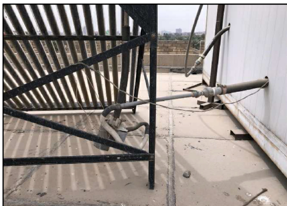
Fig. 6. The circulation pump with connection pipes.
