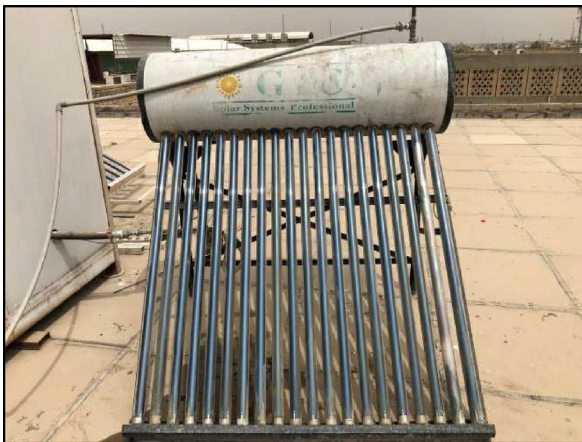
Fig. 4. An evacuated tube solar thermal collector fixed on the building roof.
